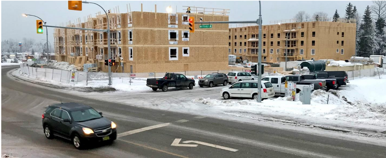
Construction of Multi Unit Residential Buildings in Prince George. Source: City of Prince George
