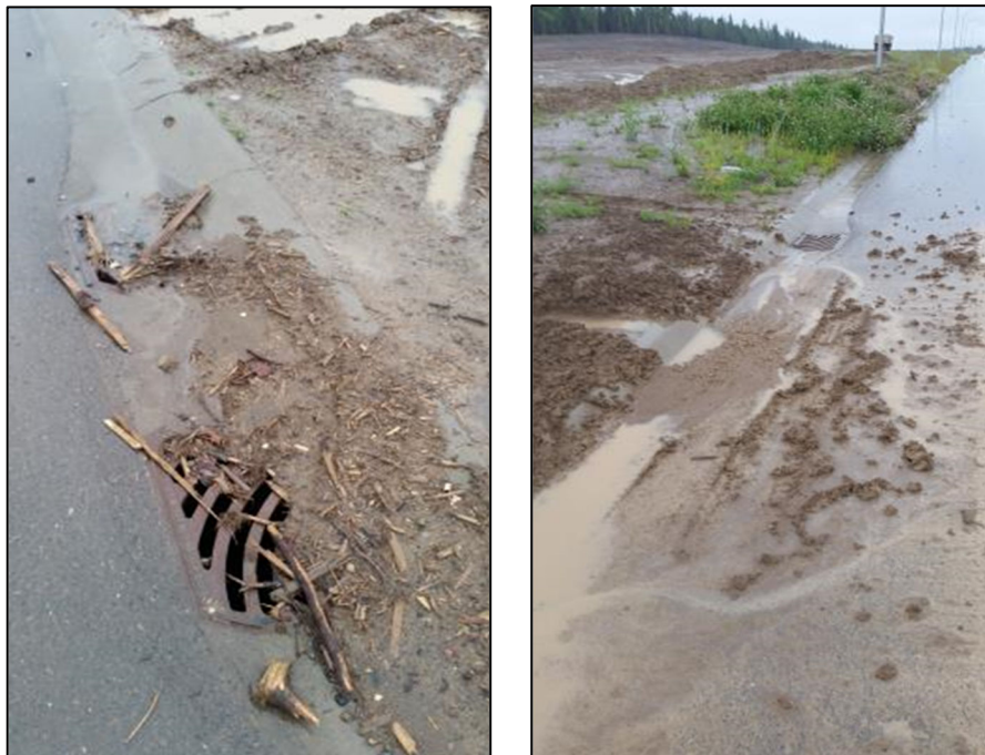
Figure 6: Erosion and Sediment
