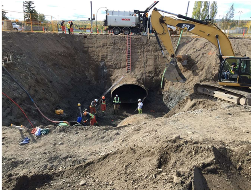
Figure 5: Winnipeg St. Sinkhole (2018) - $1.7M
