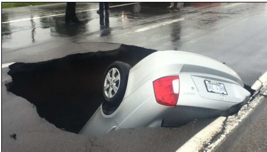
Figure 5: 2012 Sinkhole In Ottawa
