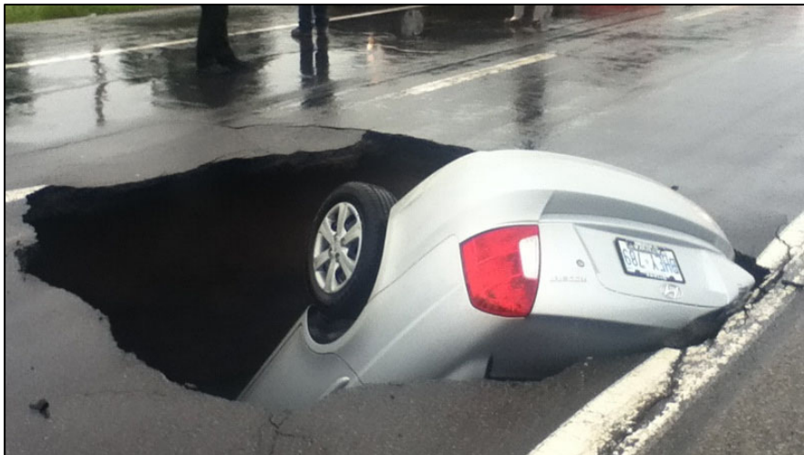
Figure 5: 2012 Sinkhole In Ottawa
