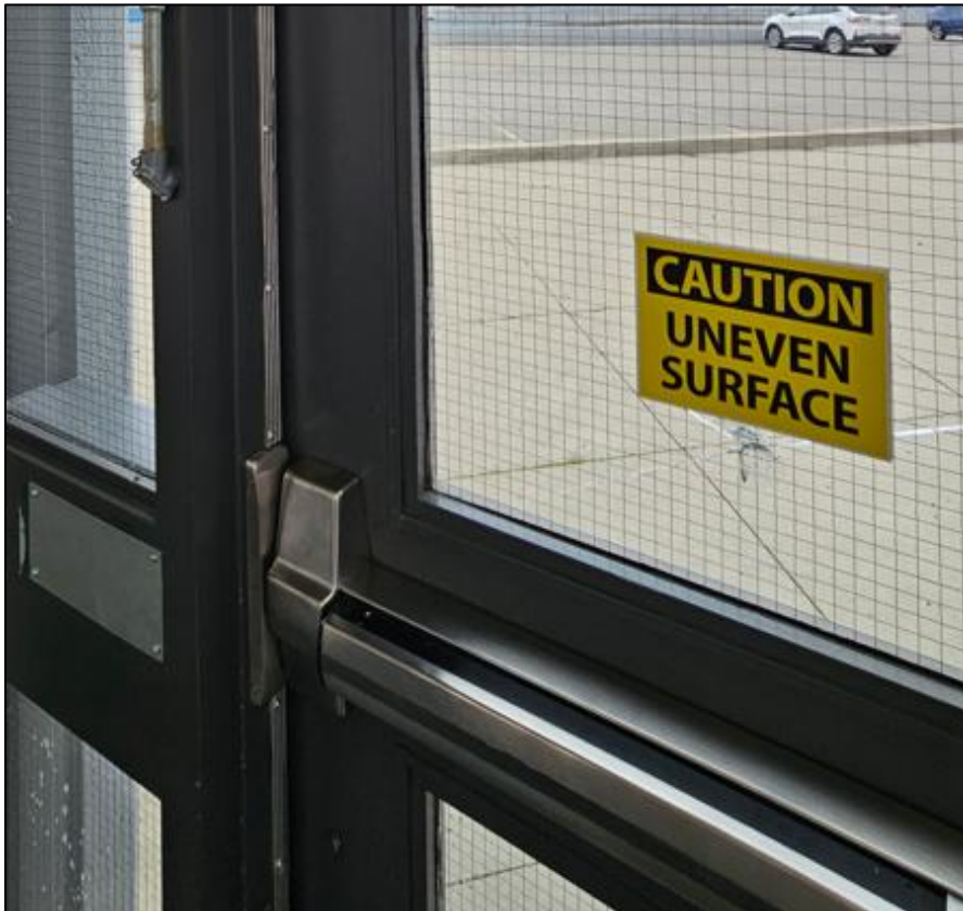
Figure 6-19: Cracked Window at Ground Level Door
