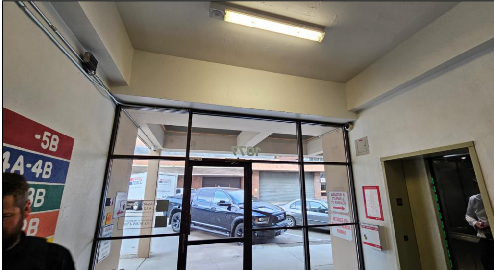
Figure 6-6: CCTV Present in P7 Plaza Parkade Lobby
