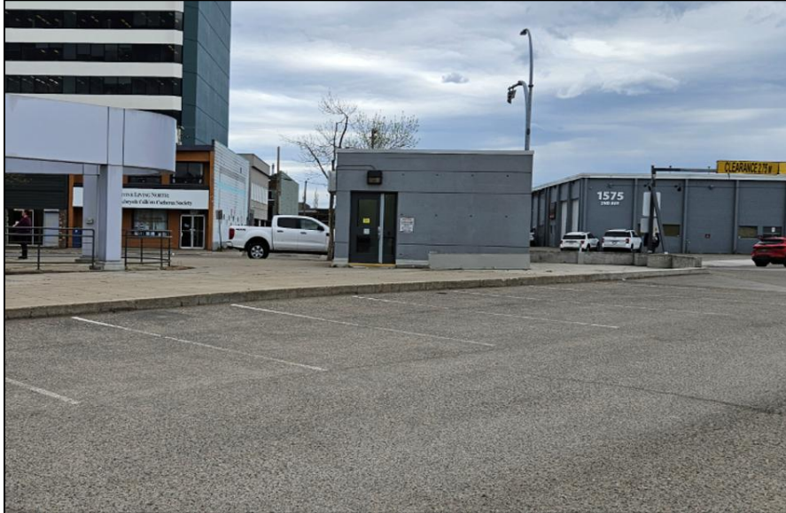
Figure 6-18: Lack of Glazing in Exterior Stairwell
