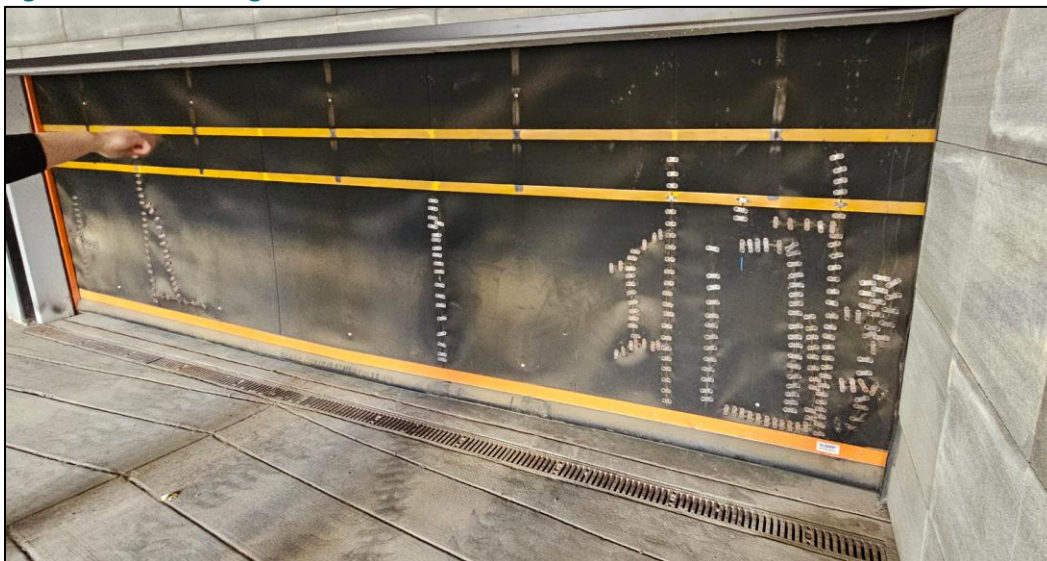
Figure 6-1: P10 George Street Parkade Overhead Door
