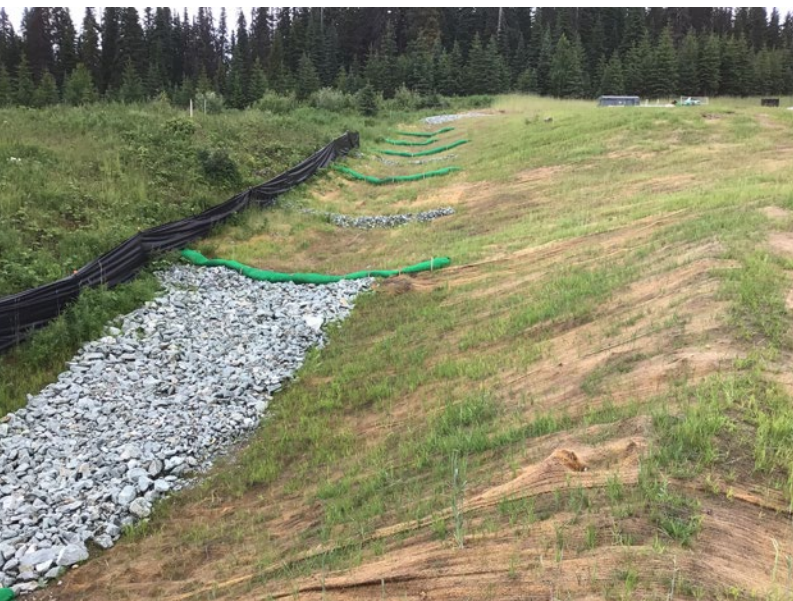
Erosion control blanket installed and showing vegetation regrowth. Rock rip rap, green waddles and sediment fencing used to manage water and sediment on site.
