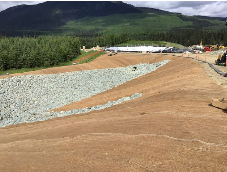
Slope lined with erosion blanket to reduce soil loss, enhance vegetative growth, and improve long-term slope stability.
