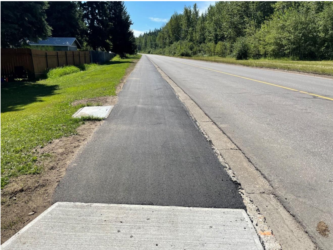
Domano Boulevard Sidewalk – Looking south from Gladstone Drive, before asphalt sidewalk rehabilitation.
