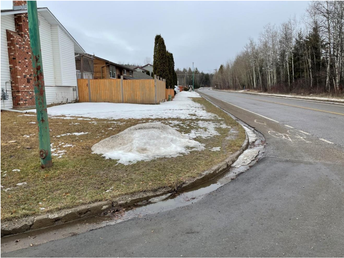
Ospika Boulevard Sidewalk – Looking west from McGowan Drive, before new sidewalk installation.
