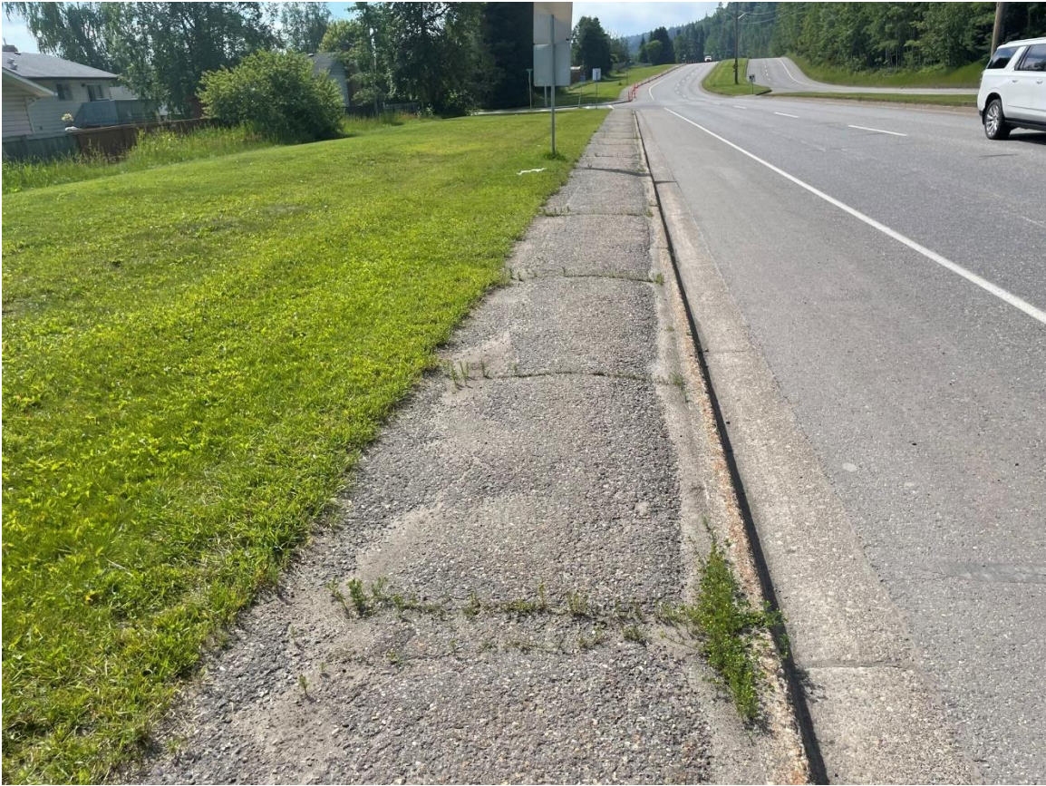
Foothills Boulevard Sidewalk - looking south towards 1 st Avenue, before asphalt sidewalk rehabilitation.
