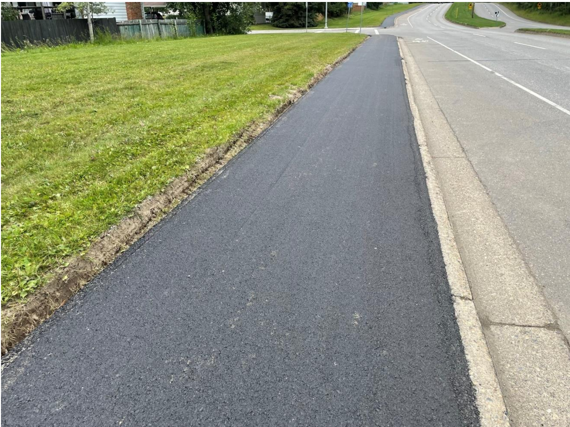
Foothills Boulevard Sidewalk - looking south towards 1 st Avenue, after asphalt sidewalk rehabilitation.
