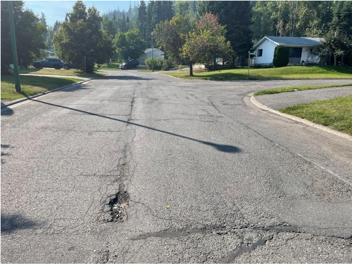
Webber Crescent – Looking south towards Rush Place, before road rehabilitation.
