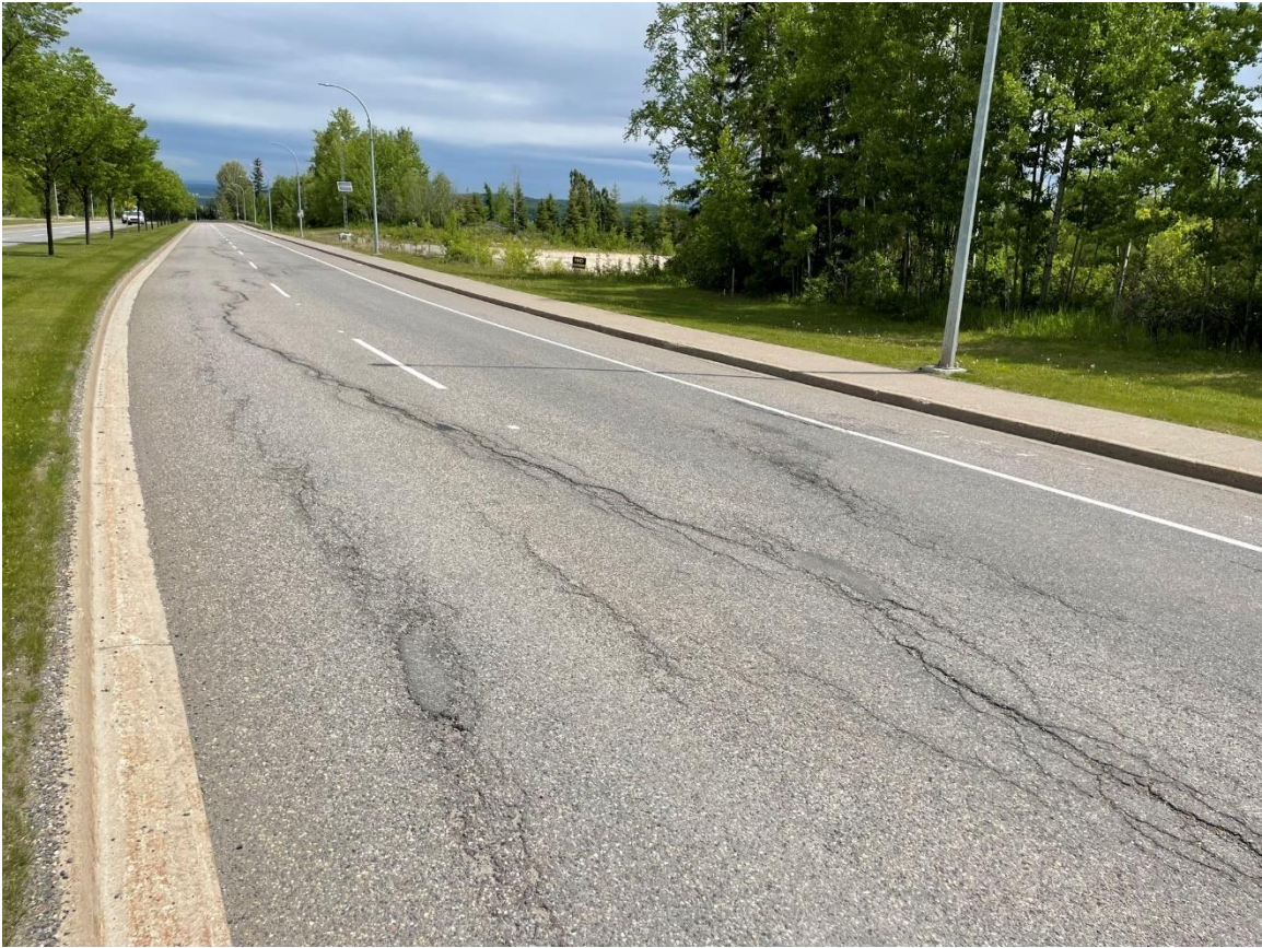
Ospika Boulevard - looking north near Tyner Boulevard, before road rehabilitation.
