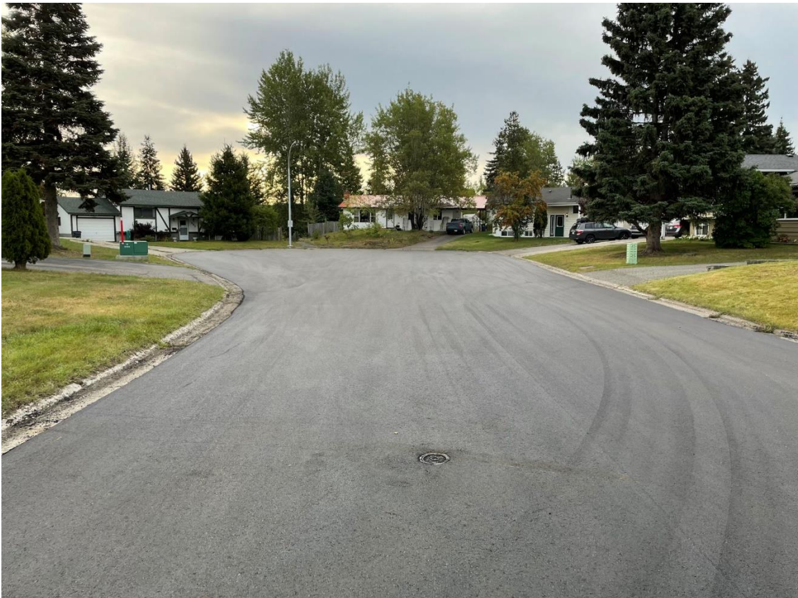
Quesnel Avenue – looking east, after road rehabilitation. The curb island was removed, and streetlight relocated to the boulevard.
