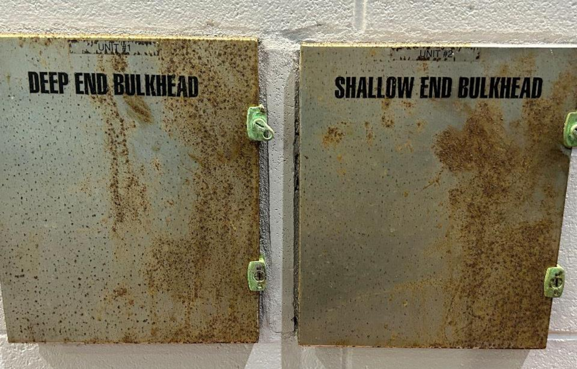
Obsolete equipment panels
