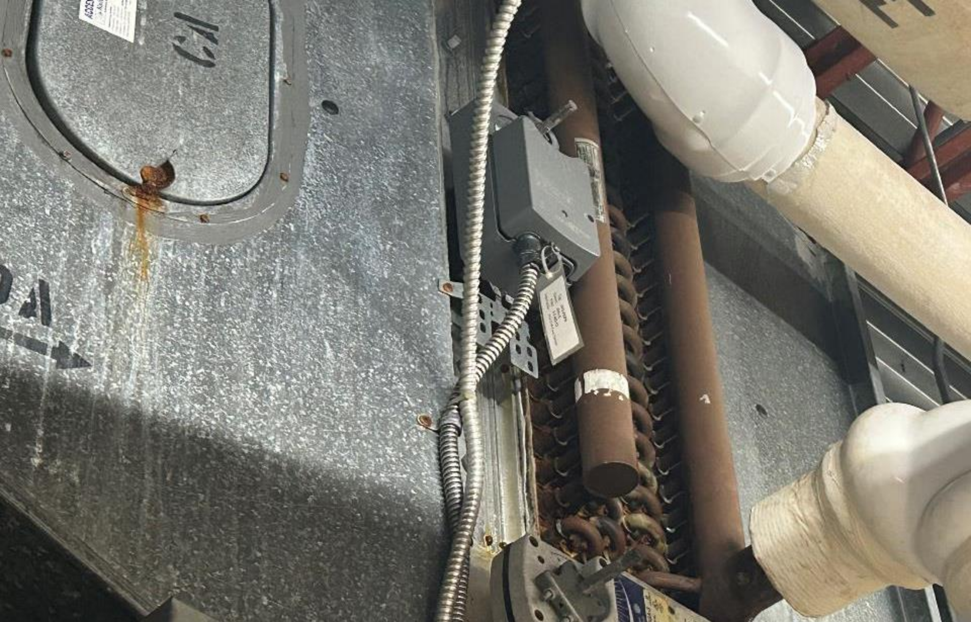
Dx Cooling coils in Air Handler
