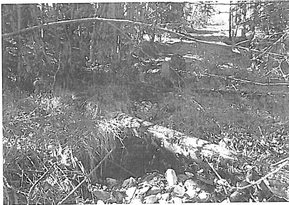
Plate 8. Tributary D, reach 1: Riprap controlled pools at outlet of storm drain pipe which forms a barrier approximately 44 m upstream of Birchwood Lake.
