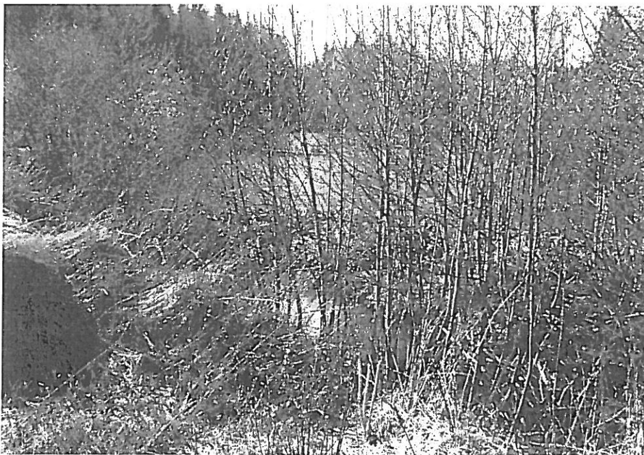
Plate 2. Tributary A, reach 1: Upstream view from above backwatered culvert inlet. Wide beaver pond in broad ravine upstream of the road grade.
