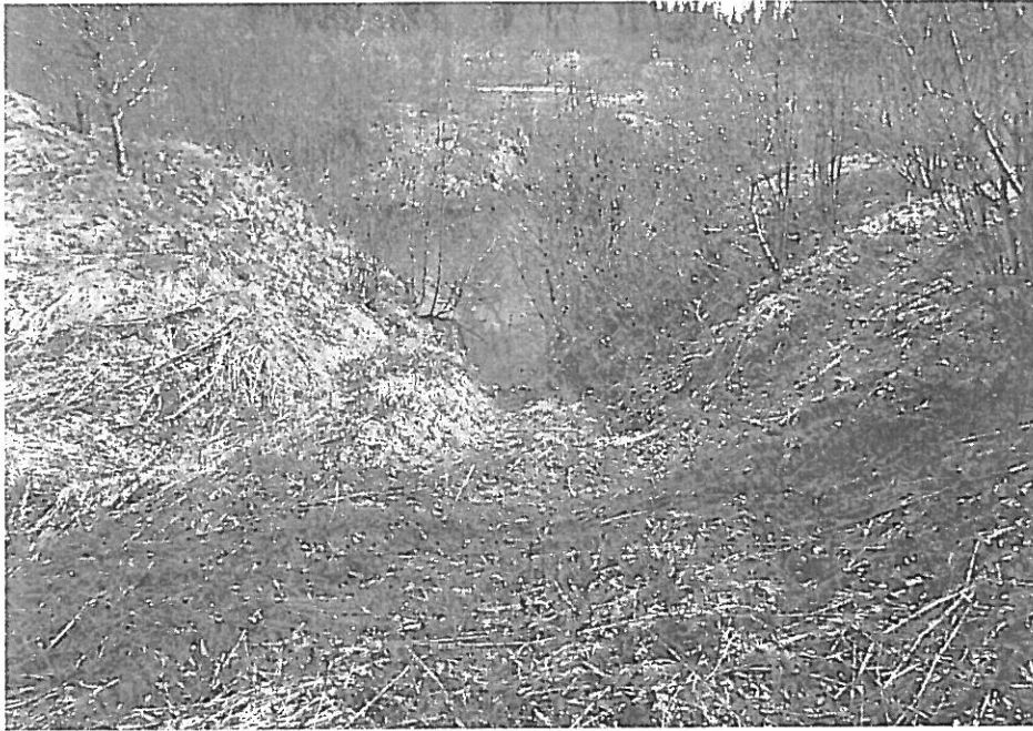
Plate 3. Tributary B, reach 1: View down ditchline toward main channel of drainage 1. An ATV ford descends the grassy slope at >30% down the embankment which forms a barrier.
