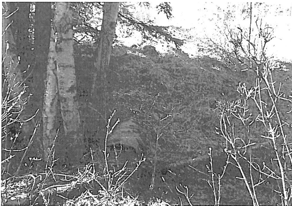
Plate 6. Tributary C, reach 2: View up drainage toward collapsed and plugged steel culvert. A NCD classification based on no defined channel. This seasonal drainage has a gradient exceeding 15% through this reach with embankment slopes exceeding 33%.
