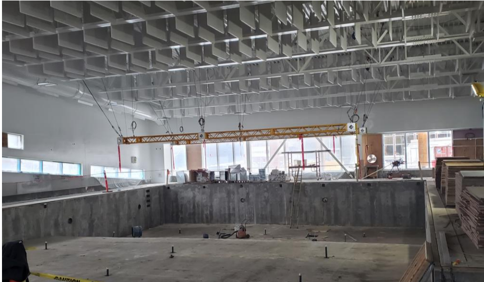
Deep pool tank with NinjaCross obstacle orange frames and white baffle ceiling above.
