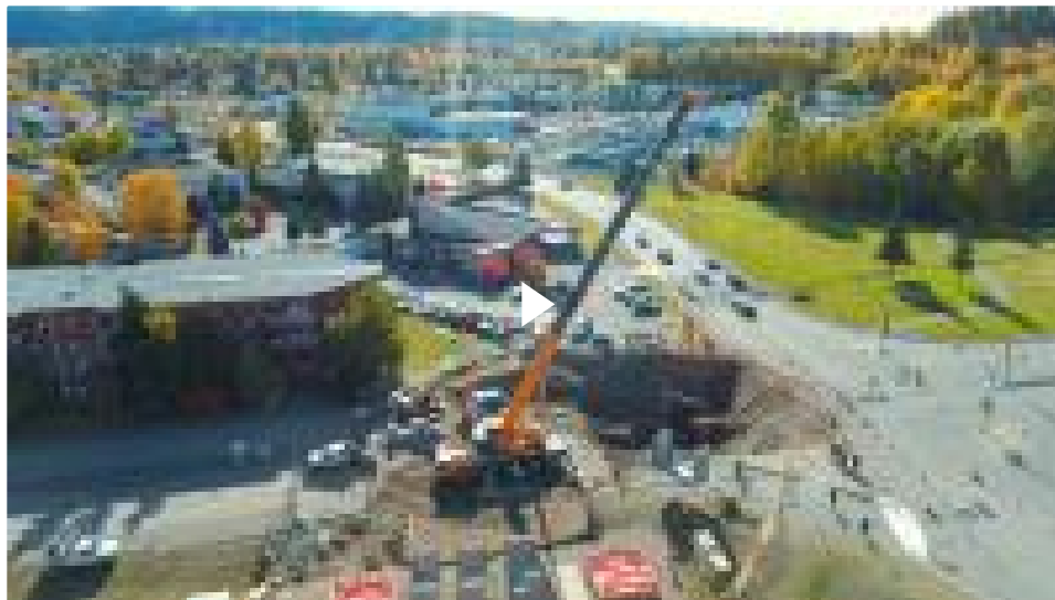
Winnipeg St. Sinkhole
